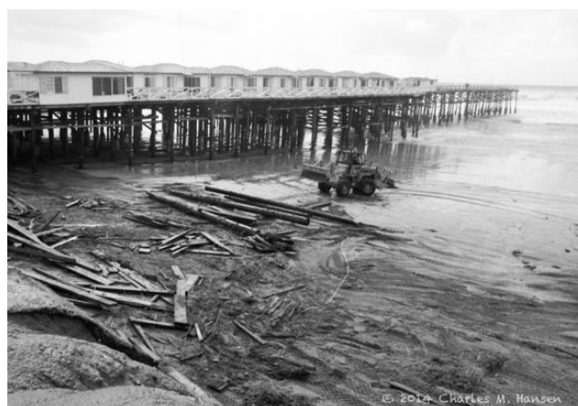
Crystal Pier Storm Damage
